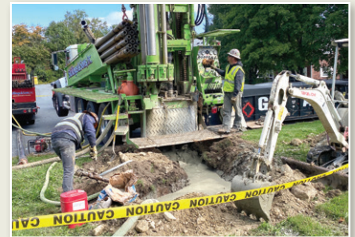
The crews conduct borehole test drilling in the Farley Lot (90 boreholes are planned throughout the route).
